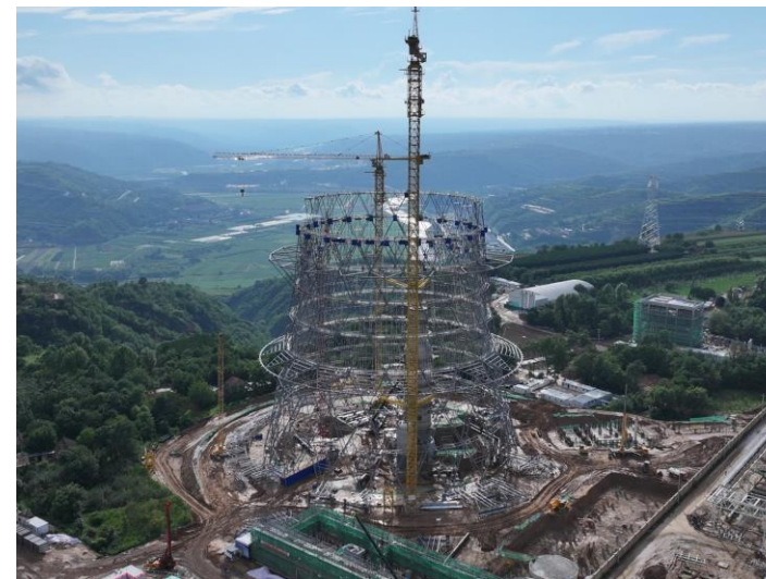
Huaneng Longdong CCUS project under construction. Image courtesy Huaneng Clean Energy Research Institute.
