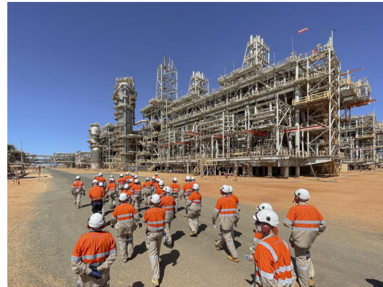
Gorgon LNG facility incorporating CCS system, Western Australia. Image courtesy of Chevron.
