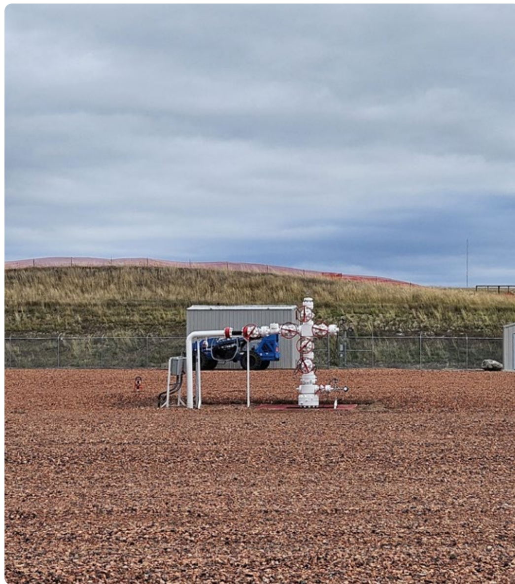
A CO 2 injection well at the Dakota Gasification CO 2 sequestration site near Beulah, North Dakota. Image courtesy Dakota Gasification Company.
