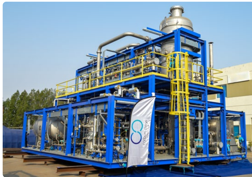
CycloneCC Industrial Demonstration Unit in the UAE. Image courtesy of Carbon Clean.
