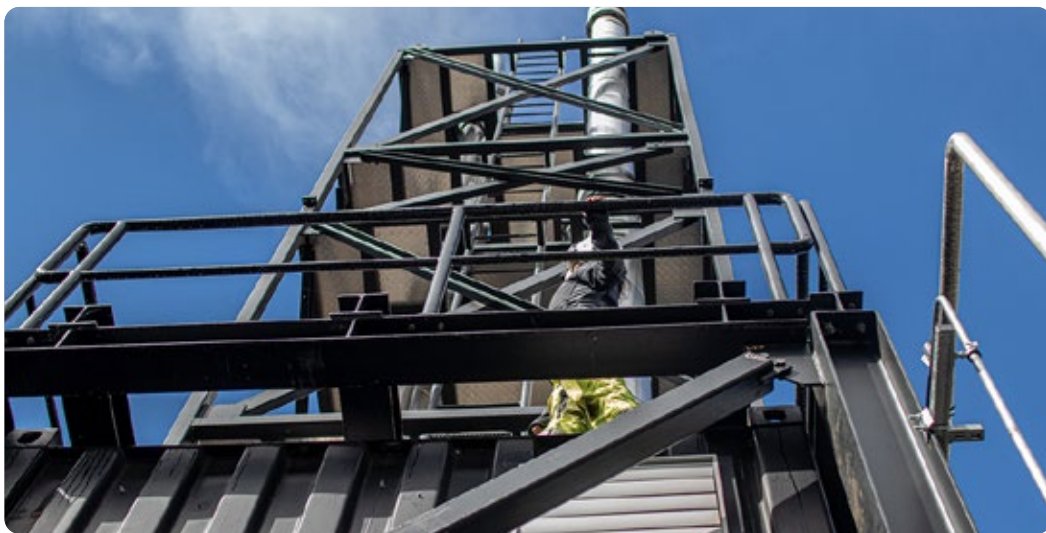
CapsolGo® at EEW Energy from Waste plant in Hanover, Germany. Image courtesy of Capsol Technologies.
