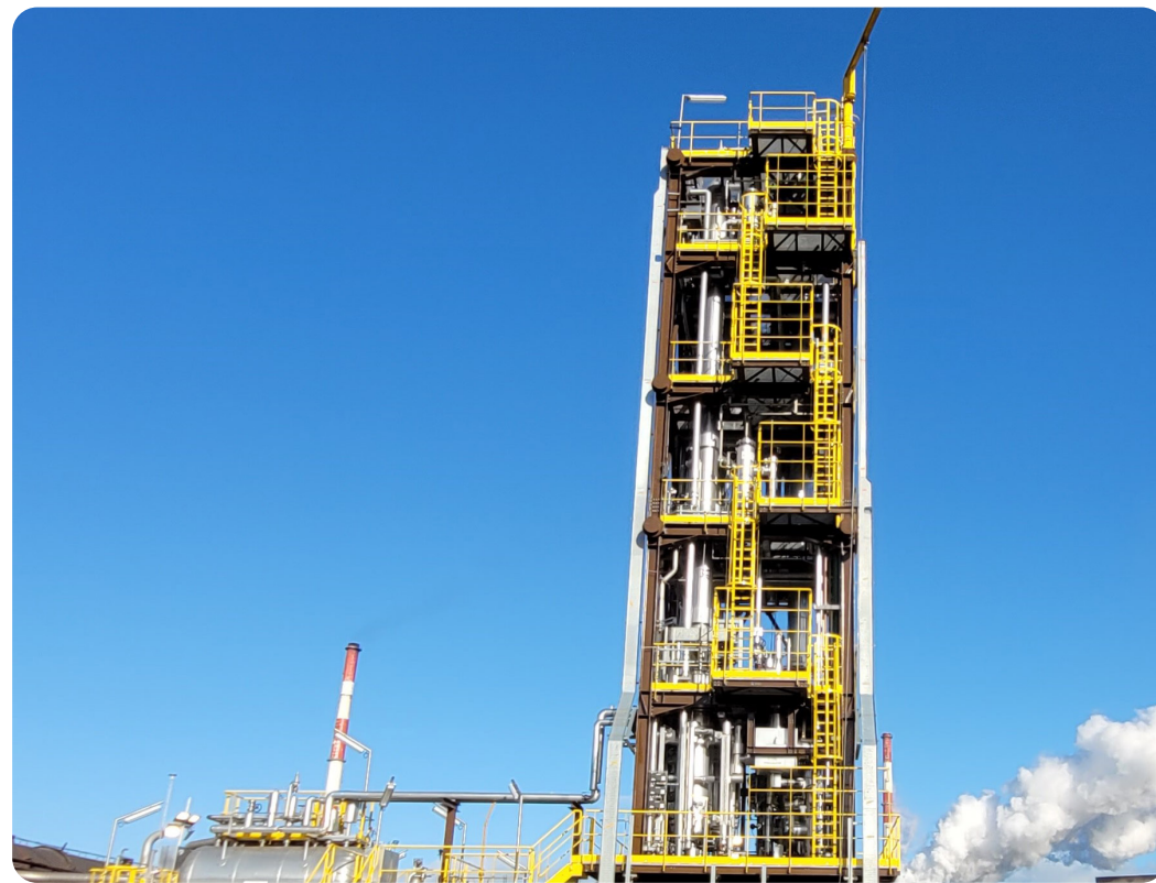
Axens DMX™ Carbon Capture Technology Demonstration plant at Arcelor Mittal Dunkirk, France. Image courtesy of Axens.
