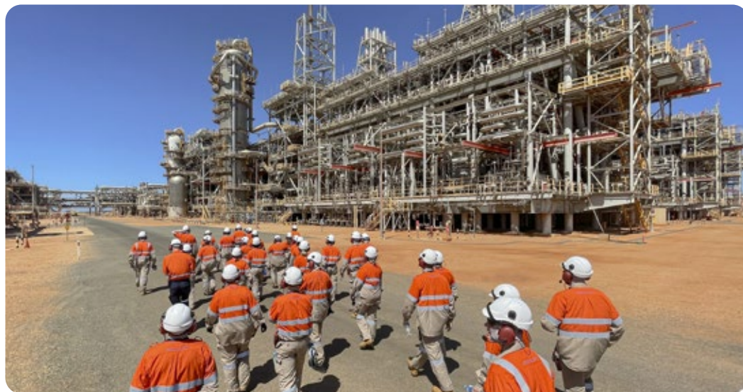
Gorgon LNG facility incorporating CCS system, Western Australia., Image courtesy of Chevron.
