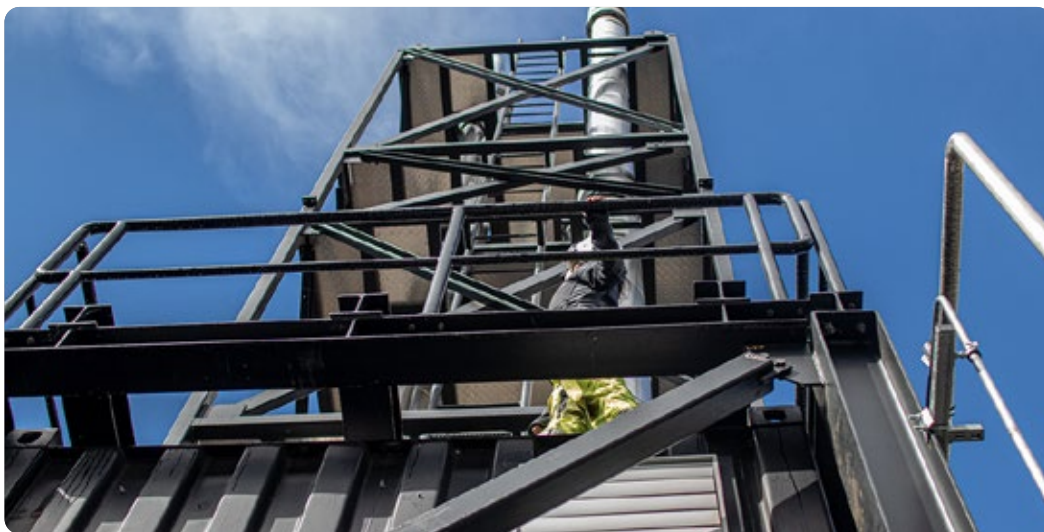
CapsolGo® at EEW Energy from Waste plant in Hanover, Germany. Image courtesy of Capsol Technologies.
