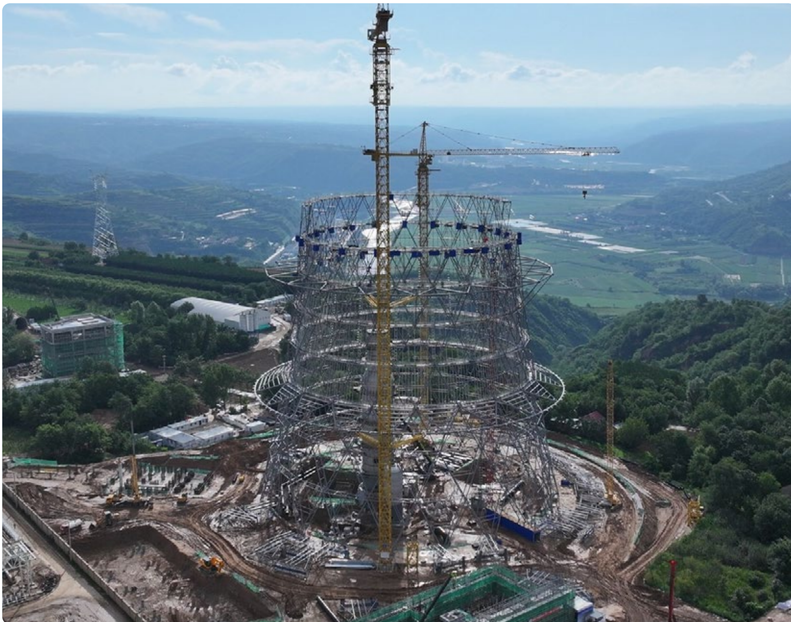
Huaneng Longdong CCUS project under construction, image courtesy Huaneng Clean Energy Research Institute
