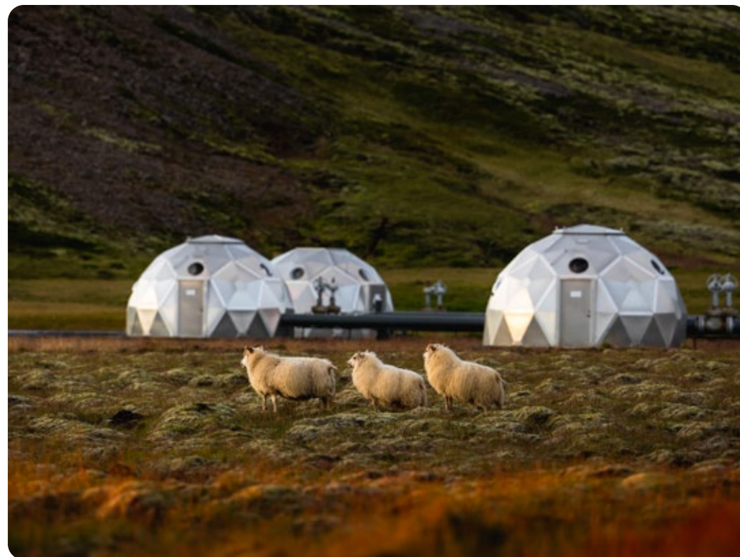
CO 2 /H 2 S Injection well in Hellisheidi, Iceland. Image courtesy of Carbfix.
