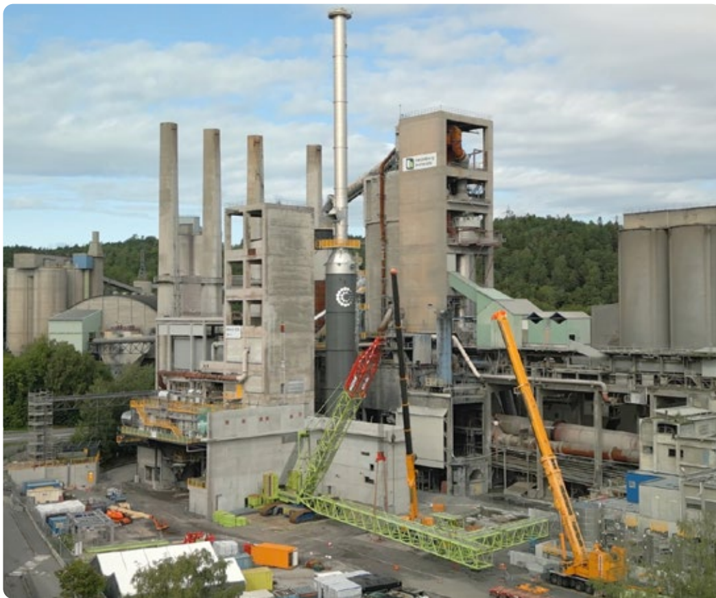
Brevik CCS facility in Brevik, Norway. Image courtesy of SLB Capturi.
