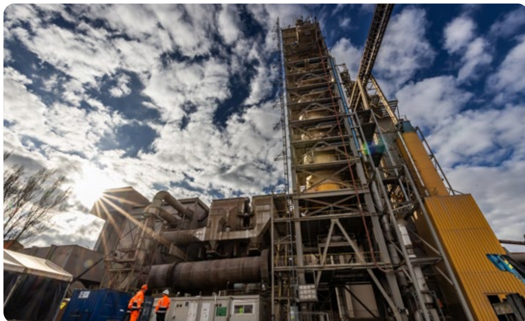
Leilac-1 Pilot Plant at the Heidelberg Materials Plant in Lixhe, Belgium. Image courtesy of Leilac Ltd.
