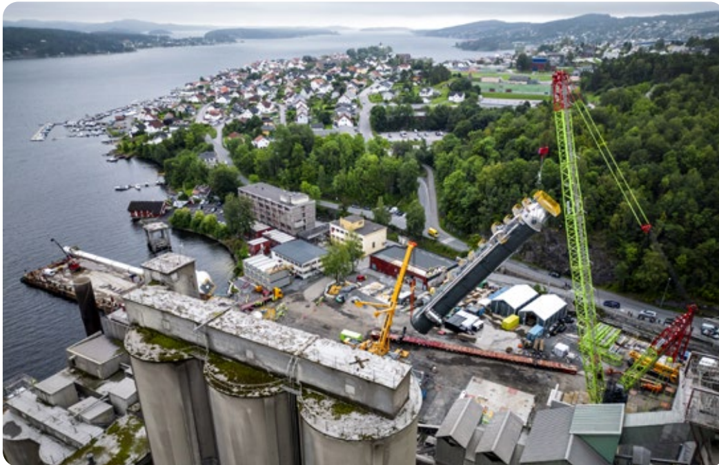
Brevik CCS facility in Brevik, Norway. Image courtesy of SLB Capturi.
