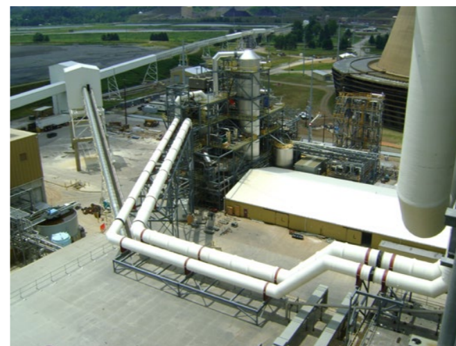
American Electric Power (AEP) Mountaineer Station
