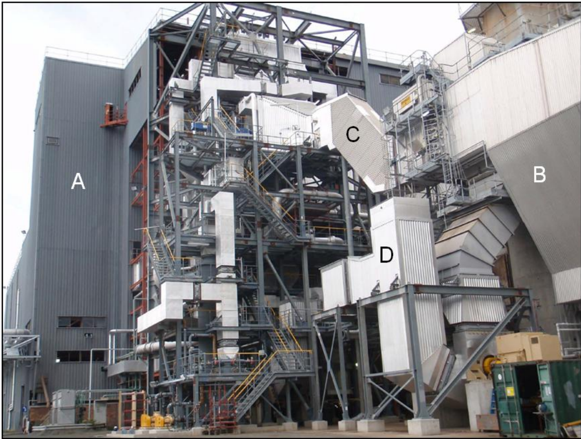
Figure 3 – View of Callide Oxyfuel Boiler equipment (A boiler house, B fabric filter, C flue gas exit duct, and D RFG duct)
