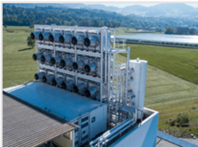
Figure 2-3. Direct Air Capture system—Climeworks.
